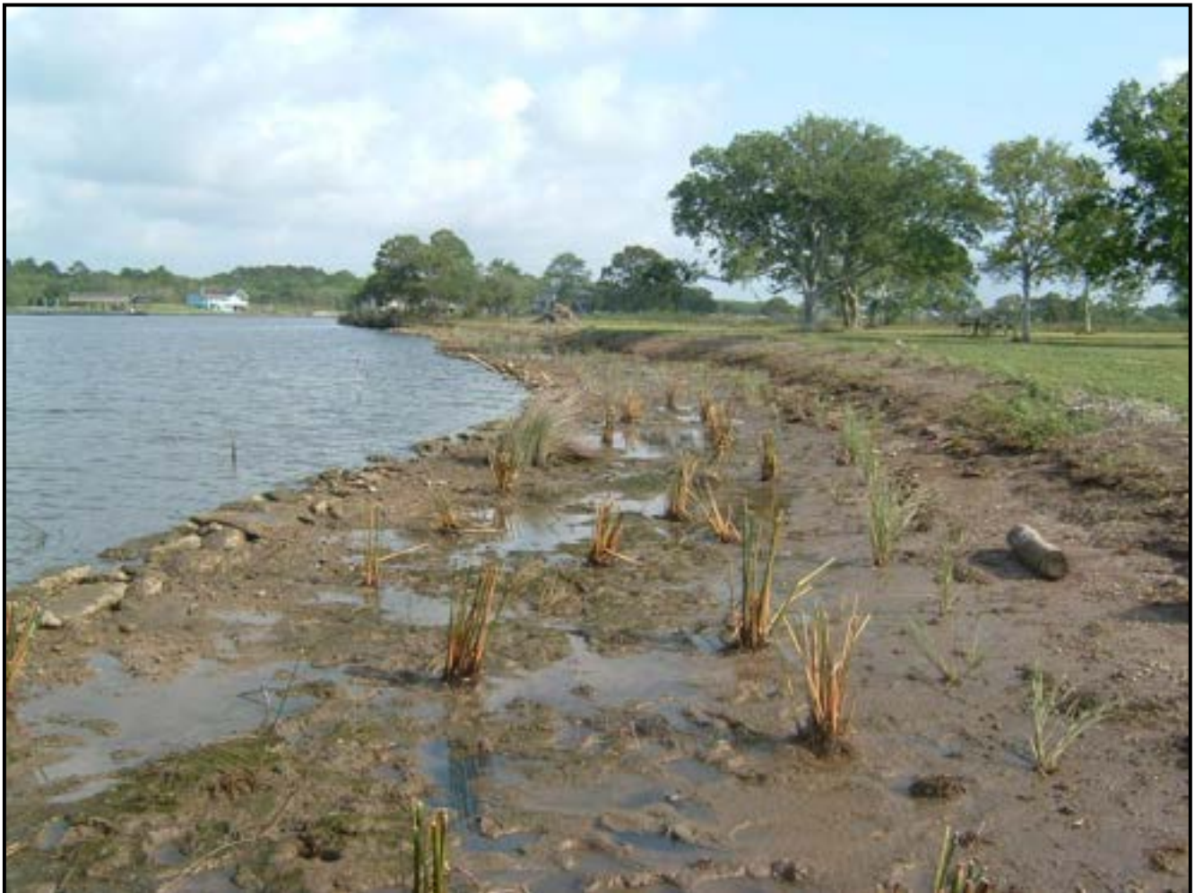
Figure 11. DURING: Planting in constructed fill area behind rock breakwater at Asher site
