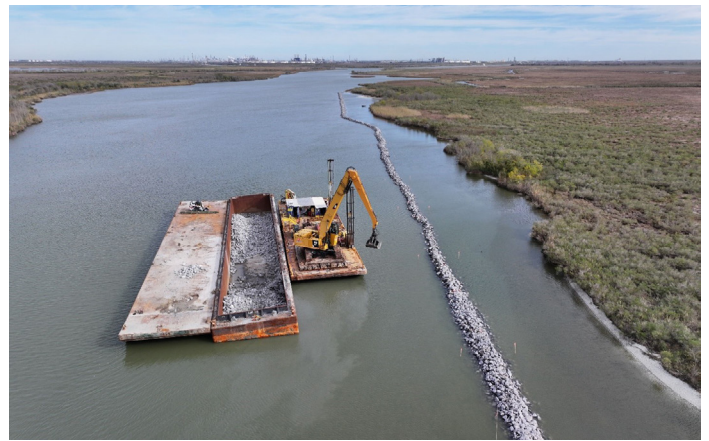
The J.D. Murphree Wildlife Management Area Shoreline Protection project constructed approximately 0.5 miles of breakwaters on the southern shoreline of the Gulf Intercoastal Waterway (GIWW) in the Salt Bayou Unit. Waves produced by boat and barge traffic in the GIWW have caused severe erosion in this area.
