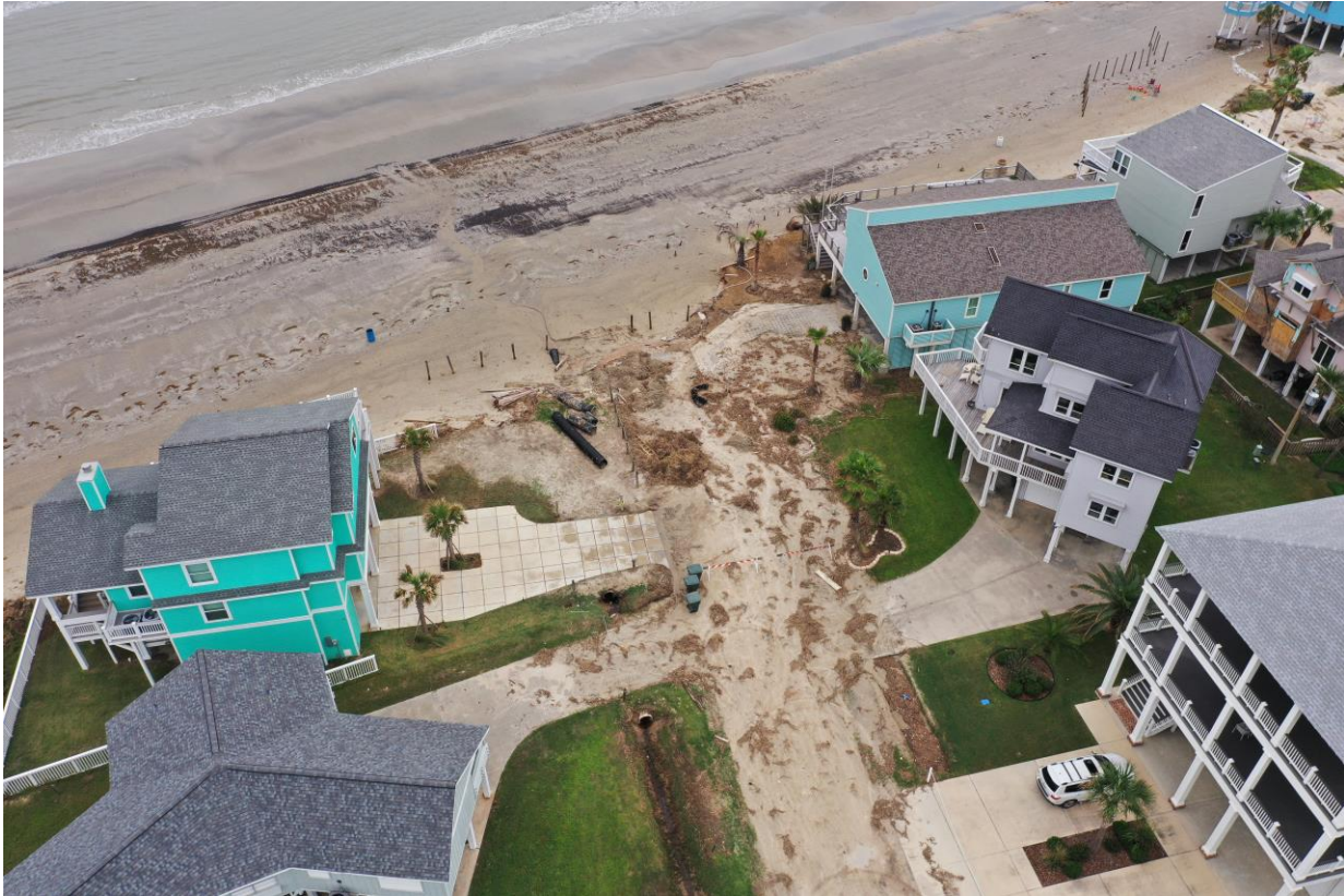
Figure 22. Drone view of the beach and access following Tropical Storm Beta (September 2020) and legacy drainage infrastructure that is collocated and affecting public beach access. (Photo courtesy: D. Henry)
