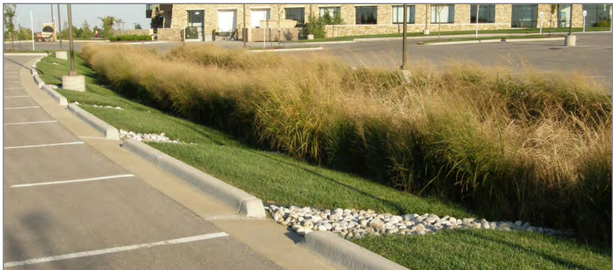
Figure 5-12: Picture of a bioretention facility. (Photo courtesy of David Dods)
