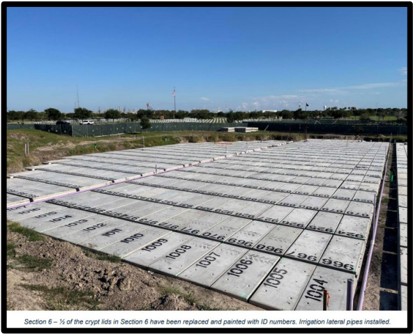
Section 6 – 1/2 of the crypt lids in Section 6 have been replaced and painted with ID numbers. Irrigation lateral pipes installed.
