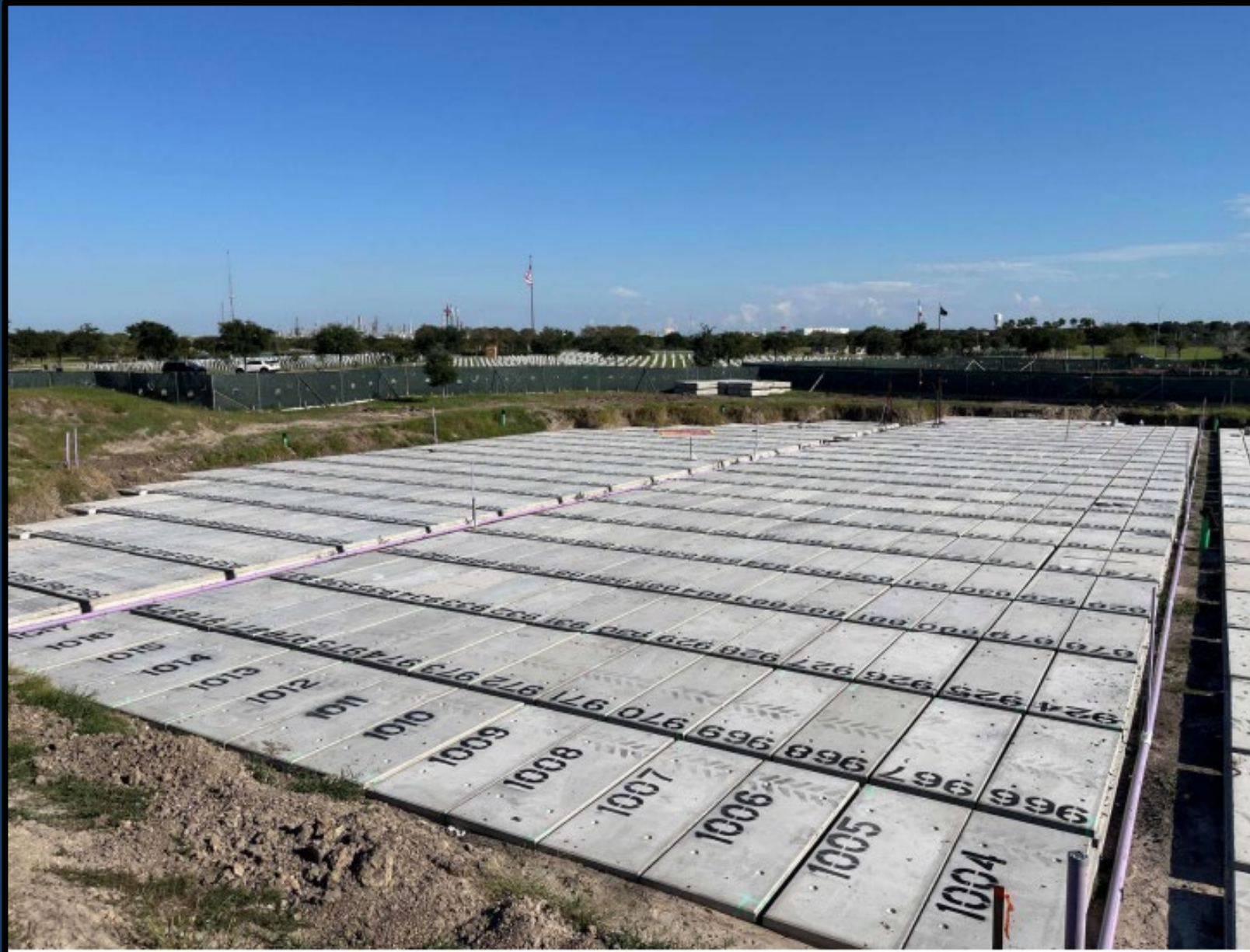
Section 6 – ½ of the crypt lids in Section 6 have been replaced and painted with ID numbers. Irrigation lateral pipes installed.
