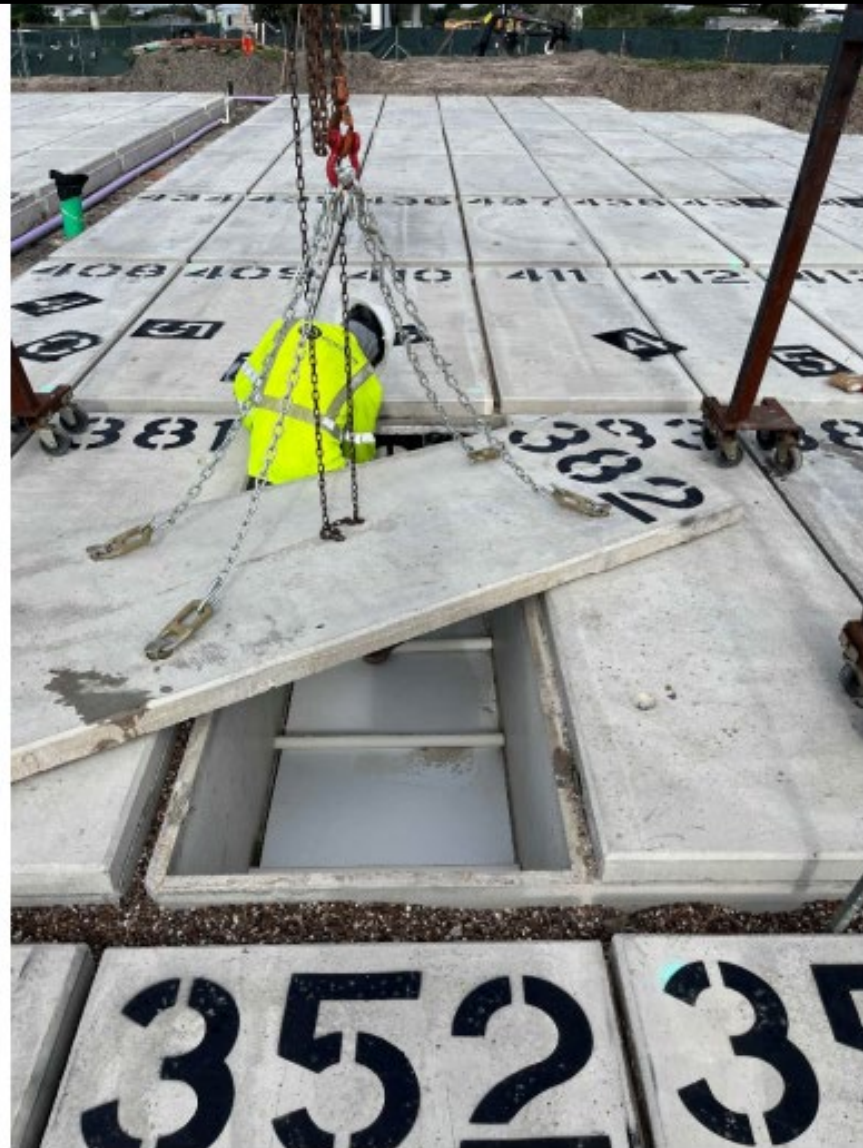
Section 7 – Removing lid to inspect crypt interior shelf and drainage slots and paint crypt ID number on interior wall.
