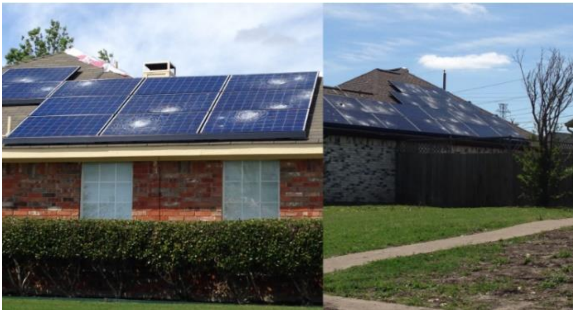
Figure 3-46: Hail damage to residential solar panels. 216
