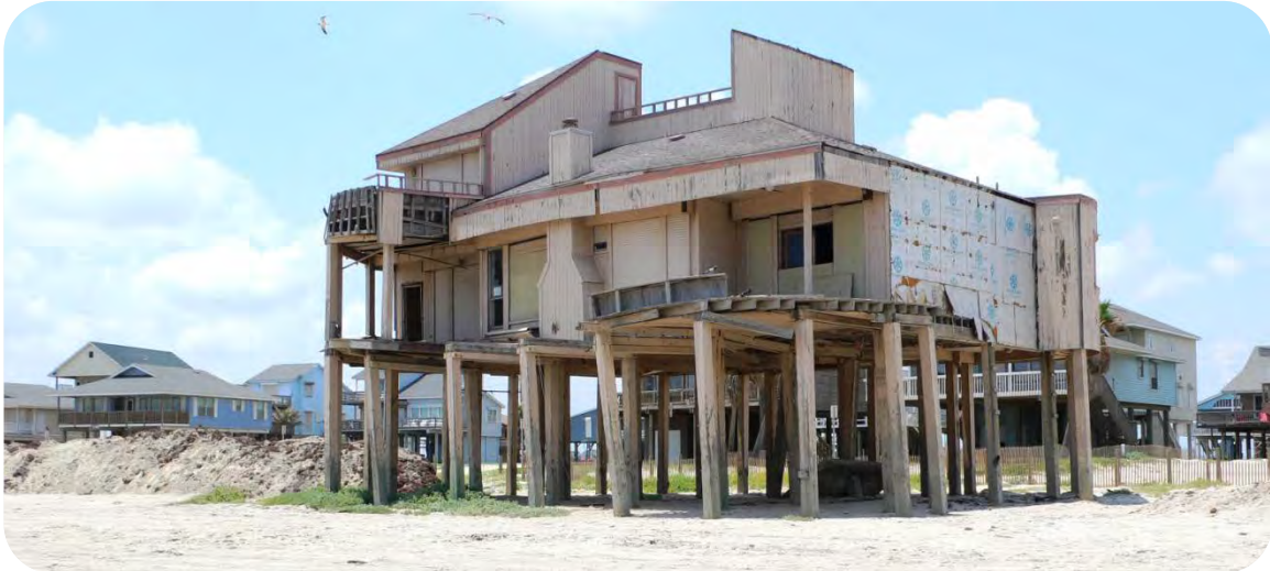
Figure 1. Effects of severe storm damage and erosion sustained during Hurricane Ike.
