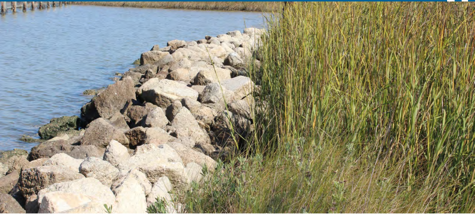
Riprap with Marsh Plants. Photo: Texas General Land Office
