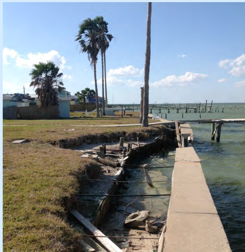
Bulkhead Failure Leads to Erosion and Land Loss Photo: Texas General Land Office
