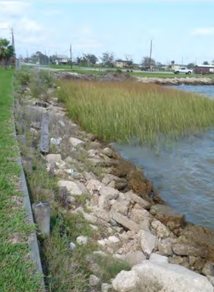
Retrofit Stabilization - Marsh Plantings with Riprap in Front of Wooden Bulkhead. Photo: Texas General Land Office
