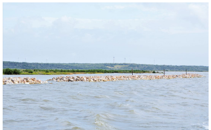
The rock rubble breakwater in Nueces Bay protects the delta’s shoreline from wave energy and erosion.
