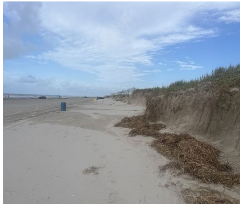
Post-Alberto (left) and post-Beryl (right) impacts to the dune system in Sunny Beach, Galveston. The GLO adopted emergency rules to allow landowners to recover rapidly from these damaging storms.
