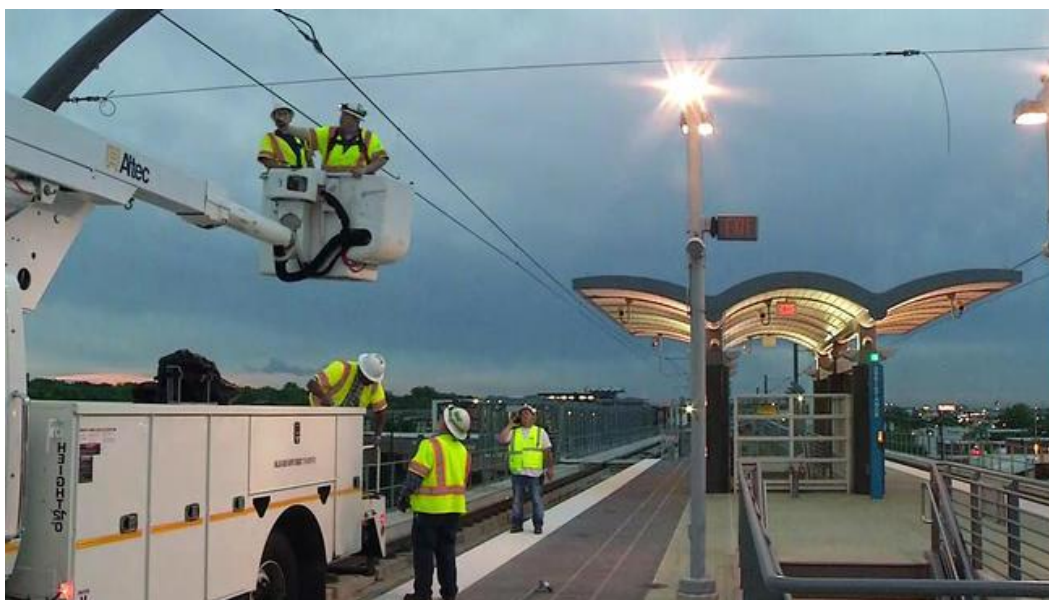
Figure 3-62: Crews work to repair the Carrollton DART rail line damaged by lightning. 345
