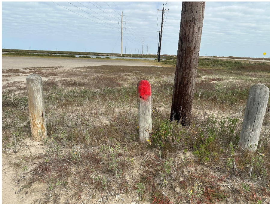
Figure 4: marked bollard to be removed/replaced
