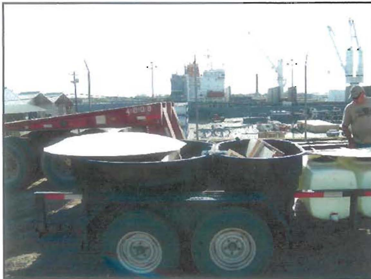
Tanks Used to Irrigate the Study Area (March 6, 2007)
