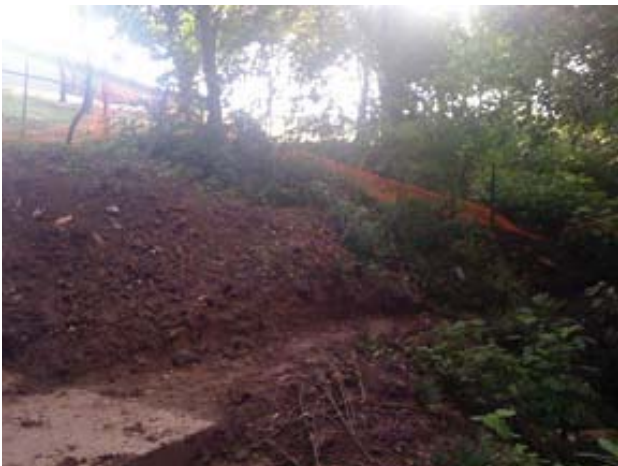
Granite step excavated and a new trail path has been configured in lieu of a stair because of steep slope.
