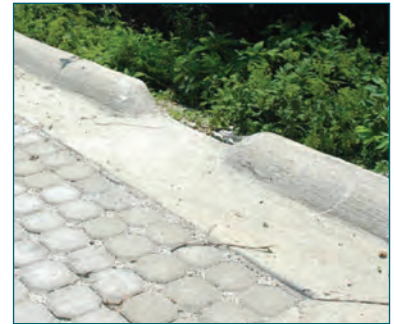
Figure 4. Curb cut opening. (Source: USDA, NRCS)
