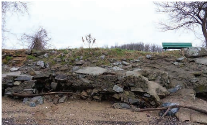
Undercutting of the Gambacorta Marsh Dike in New Castle, Delaware, as shown here is just one of the problems faced by dikes in Delaware's coastal zone. Credit: DNREC
