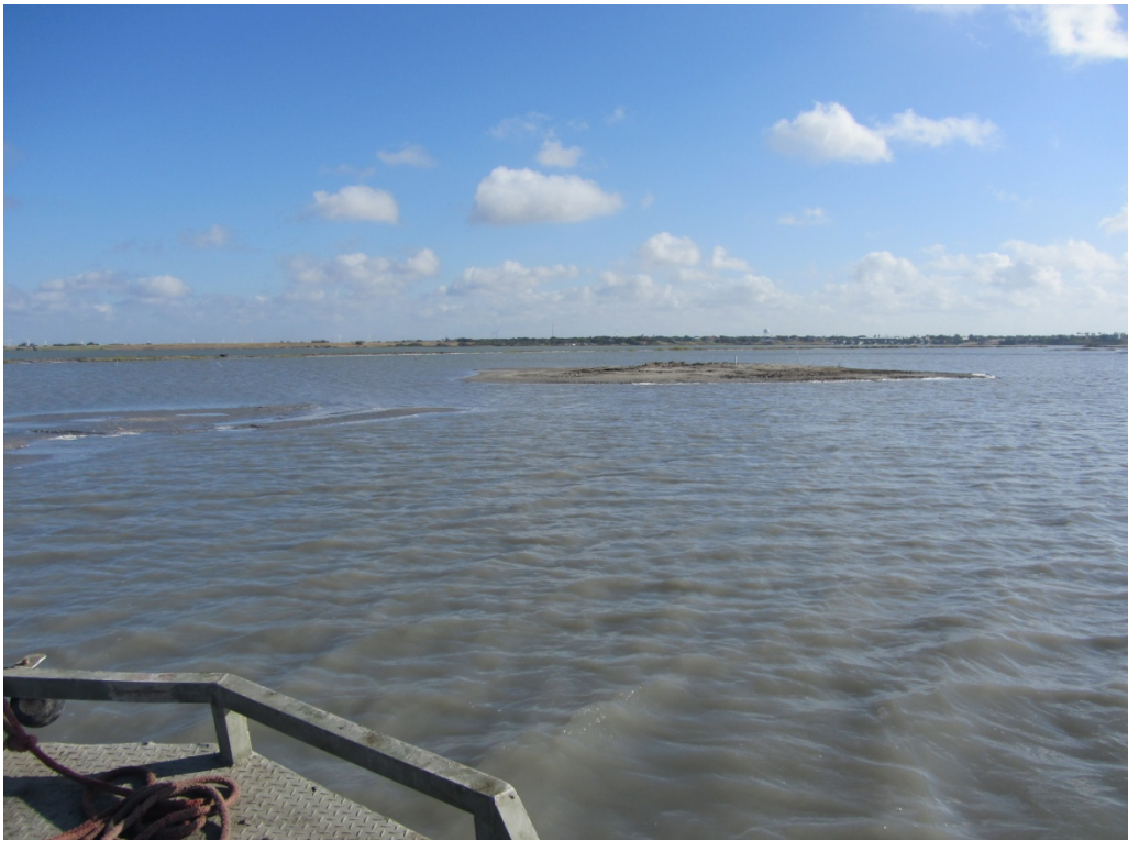
Material placed between M2 and M3. M3 shown and newly placed material on the left.
