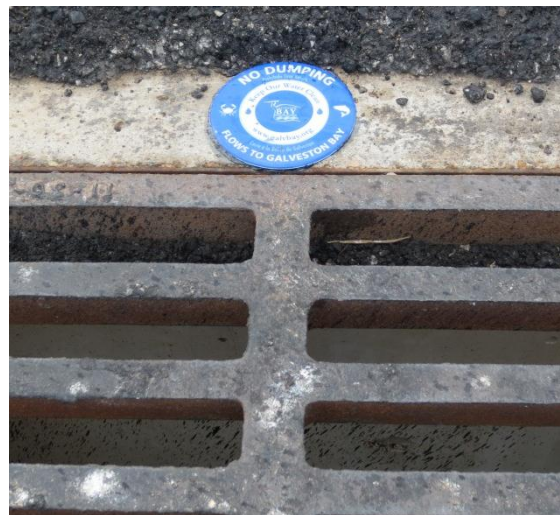
Figure 22. Storm drain markers installed at Pelican Rest Marina
