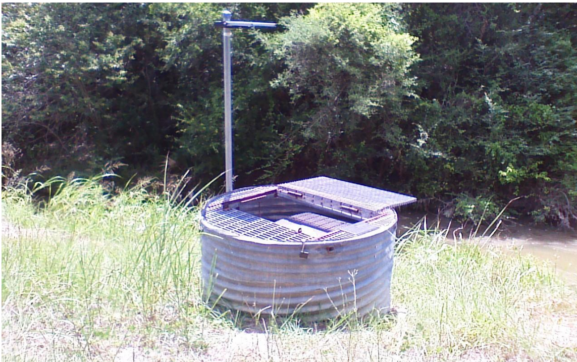
Figure 6. Manhole used for equipment storage and runoff collection at the OSSF site.
