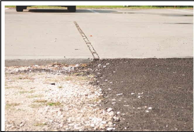
Entrance to Palmetto Avenue parking area. The difference in height between the gravel surface and the concrete surface and the street was not ADA compliant, so the county contracted for construction of an asphalt section so the entrance from the street would be smooth.
