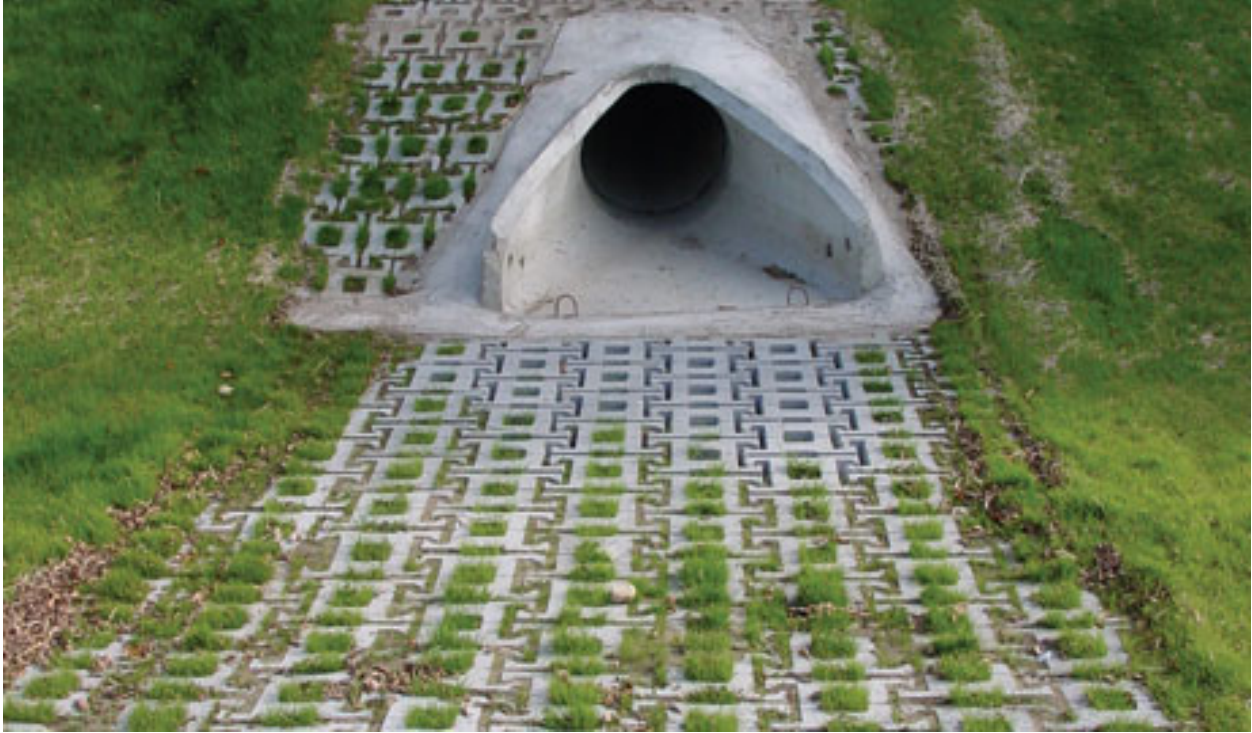
Figure 3. Photo of Armorflex structure installed to prevent further creek bank erosion and promote the growth of existing habitat.
