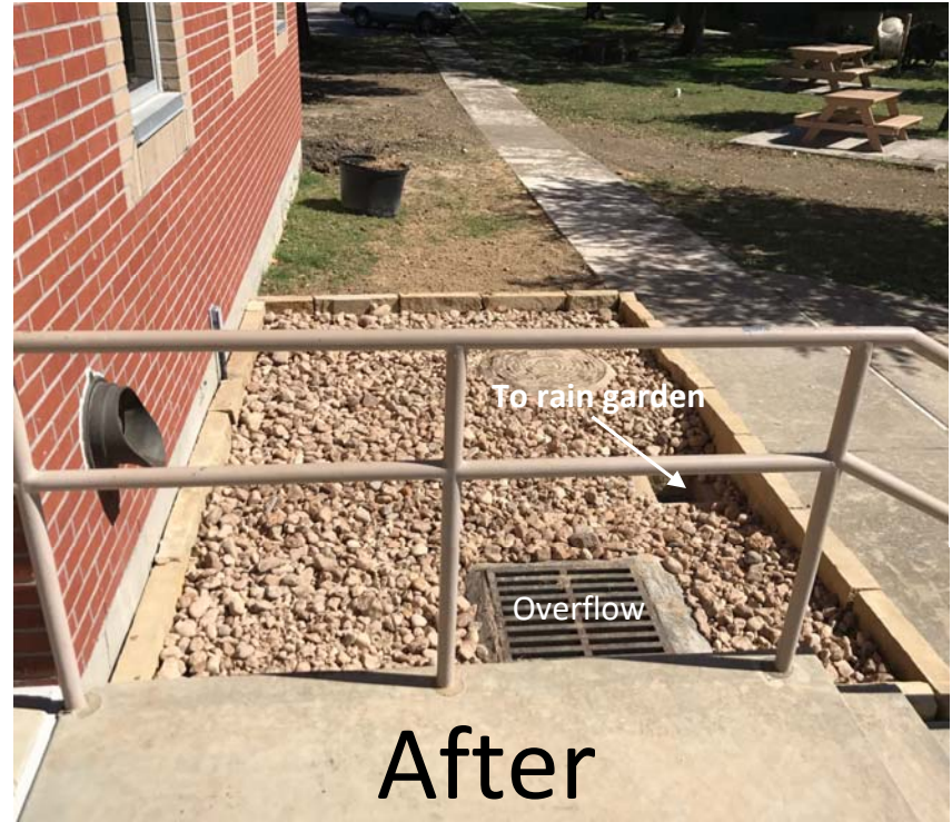
City of Pasadena staff designed and installed the rock basin as part of the rain garden system. Water fills the rock area then drains first into the basin on the right into pipes connected to the rain garden. During large rainfalls, the large storm drain serves as an overflow so the area does not flood.
