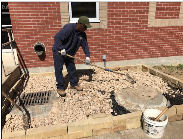
New ponding/drainage area by the building, the pipes under the sidewalks begin here
