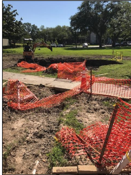
Installation of pipes under two sidewalks to move water from the down spout into the rain garden
