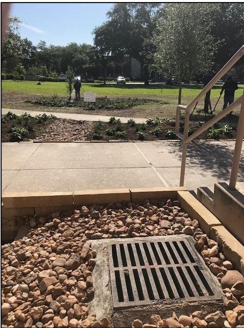
View from the down spout on the library, you can see the drainage structure in the foreground, WaterSmart garden in the middle, and rain garden in the back.
