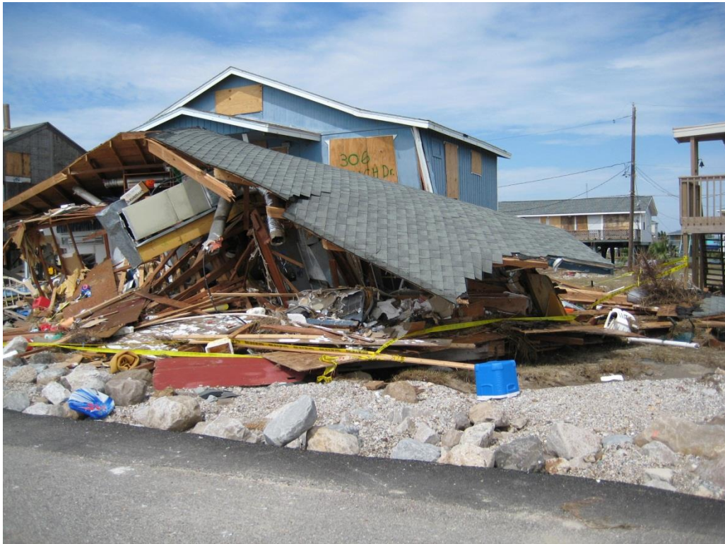
Figure 3.15 Home damage in Surfside, TX.
