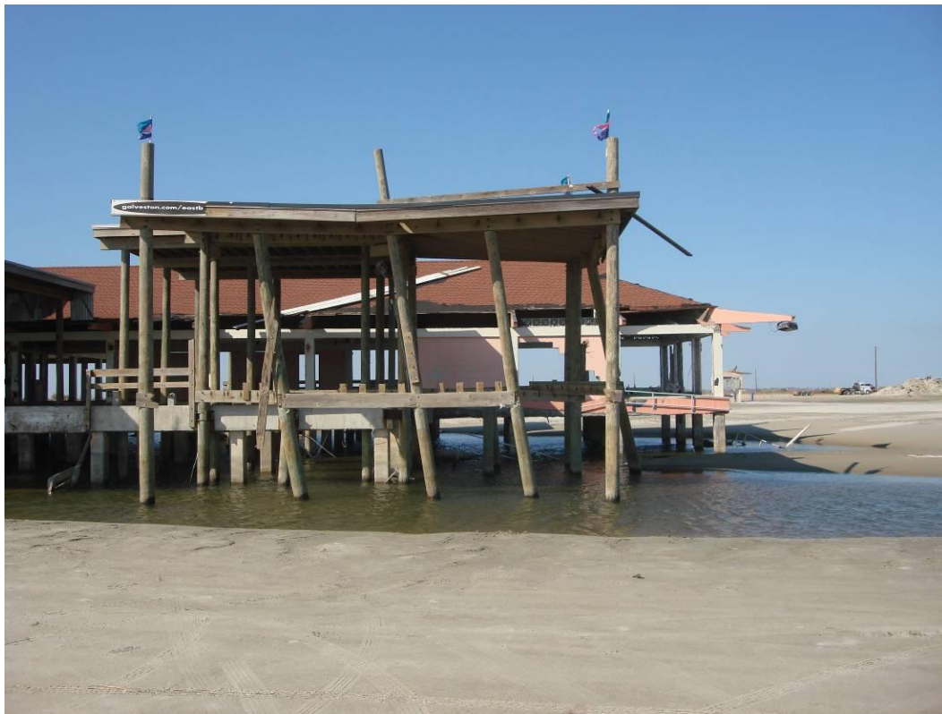
Figure 3.7 Pavilion on East Beach damaged during Ike.
