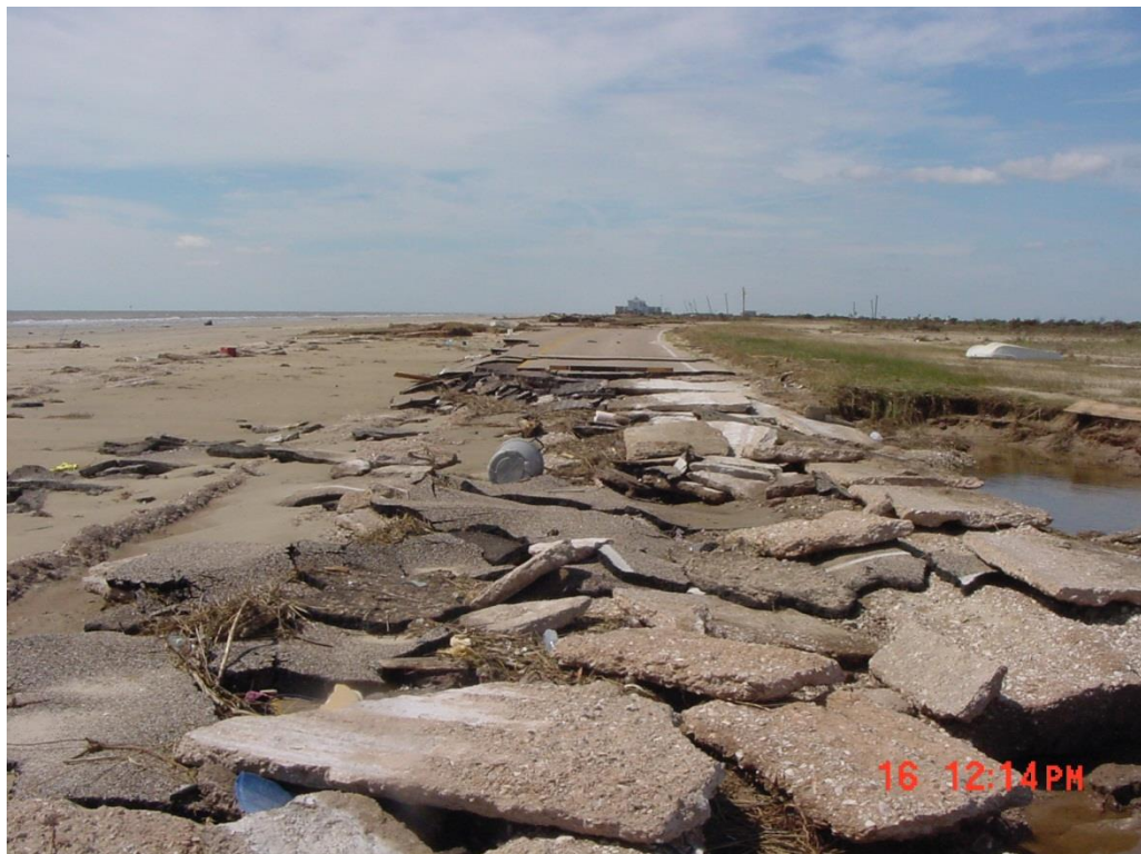
Figure 3.16 Damage to Blue Water Highway on Follets Island.
