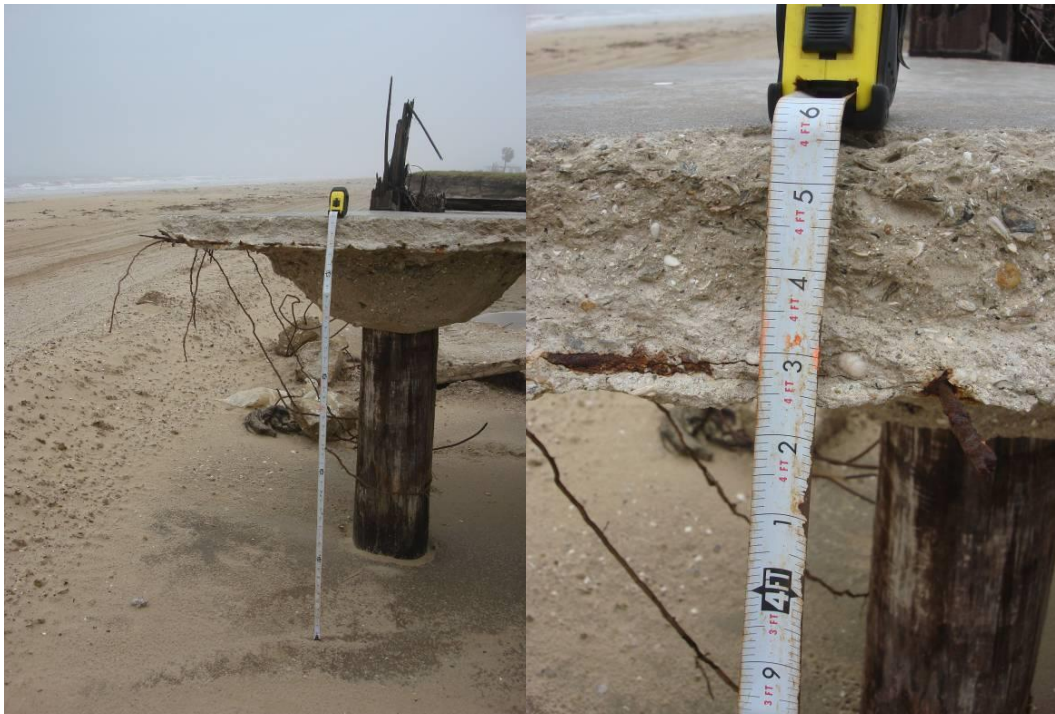
Figure 3.3 Erosion under a house foundation south of Rollover Pass.
