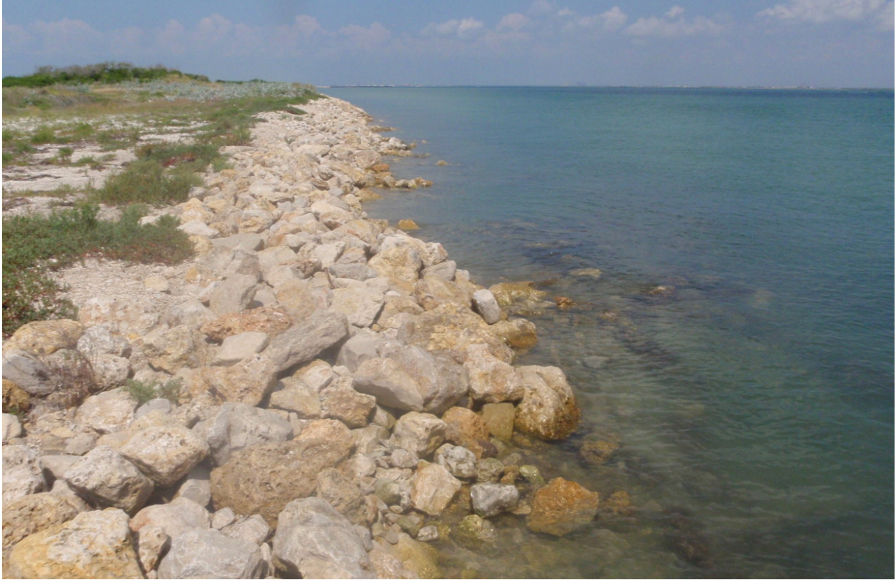
Figure 4.2 Revetment Repair Project Pre-construction Conditions (6/28/12; photo provided by GLO)
