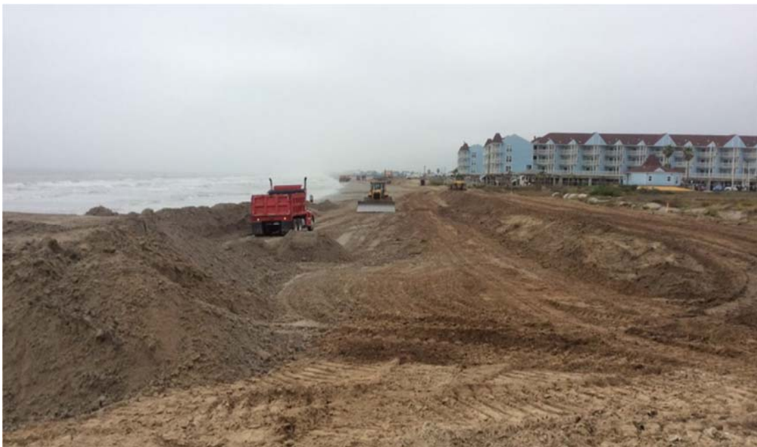
Figure 3.1.3 Construction of the end of seawall beach nourishment (12/4/14; Photo provided by GLO)
