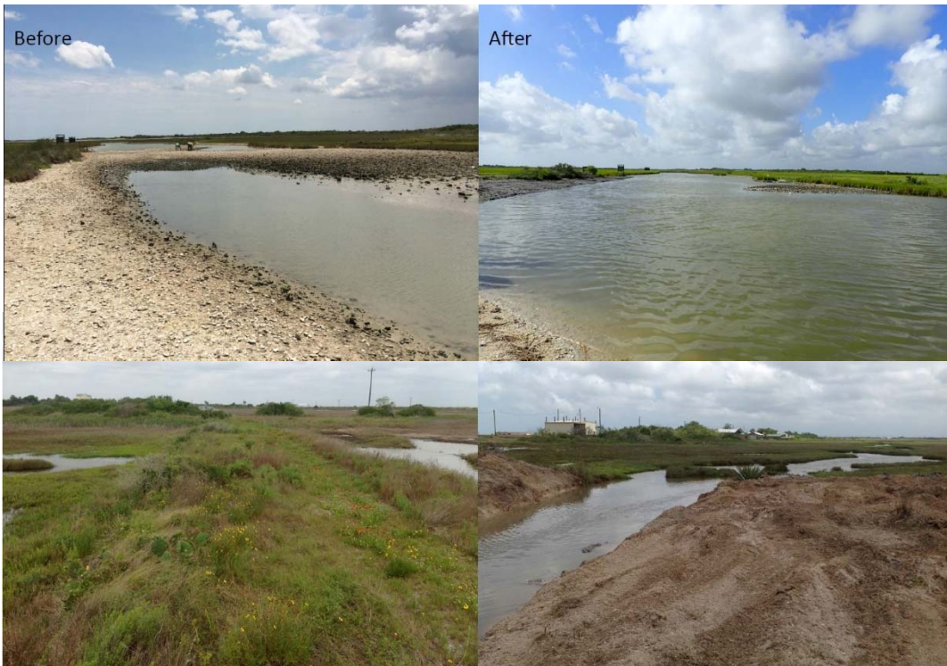
Figure 4.7.2 Magnolia Inlet Before and After Removal of the Shoal Blocking Tidal Exchange (Photos from Feagin (2016))
