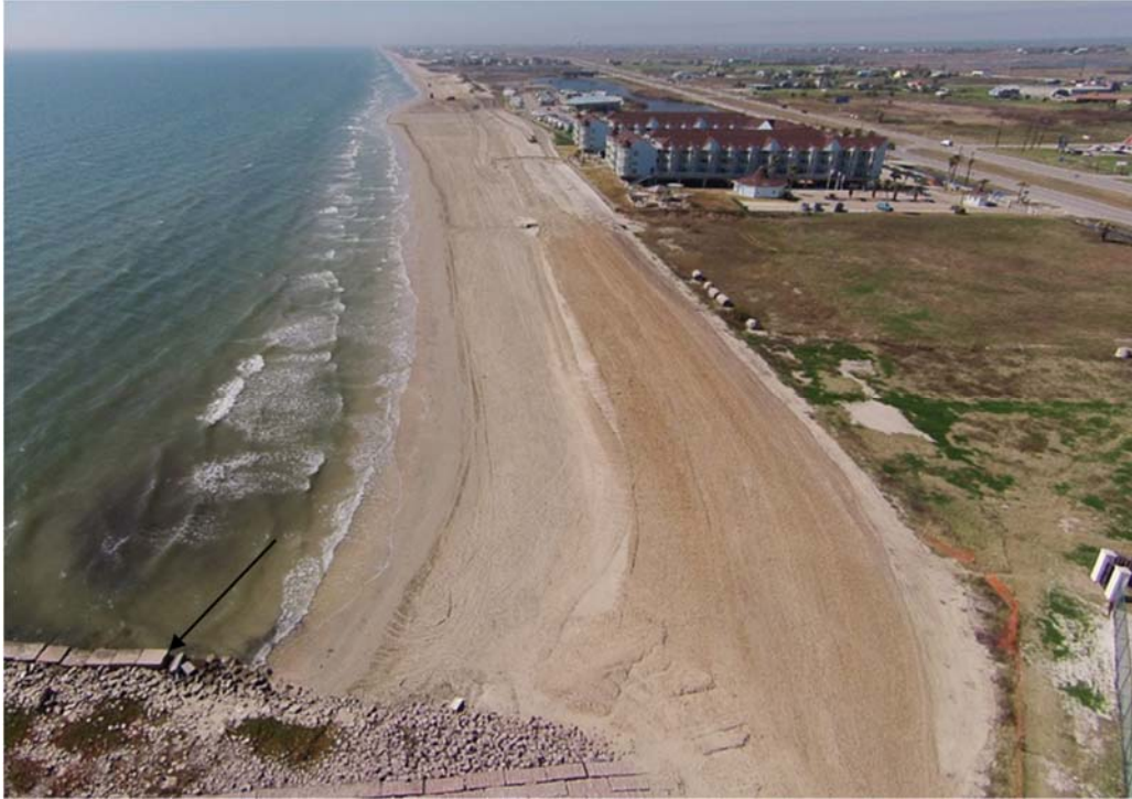
Figure 3.1.4 End of seawall beach nourishment near the construction completion (around March 2015; Photo provided by GLO) (The arrow shows a point of reference also displayed in Figure 3.1.2)
