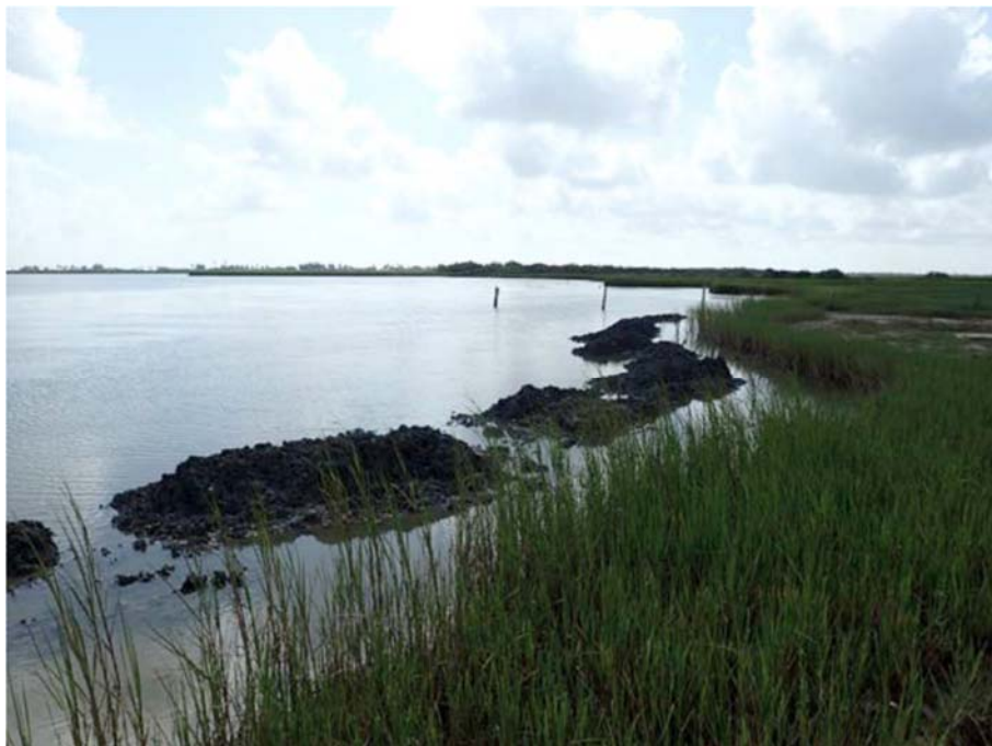
Figure 4.7.3 Shore Protection Measure on the South Side of Old Town Lake. (Photo from Feagin (2016))
