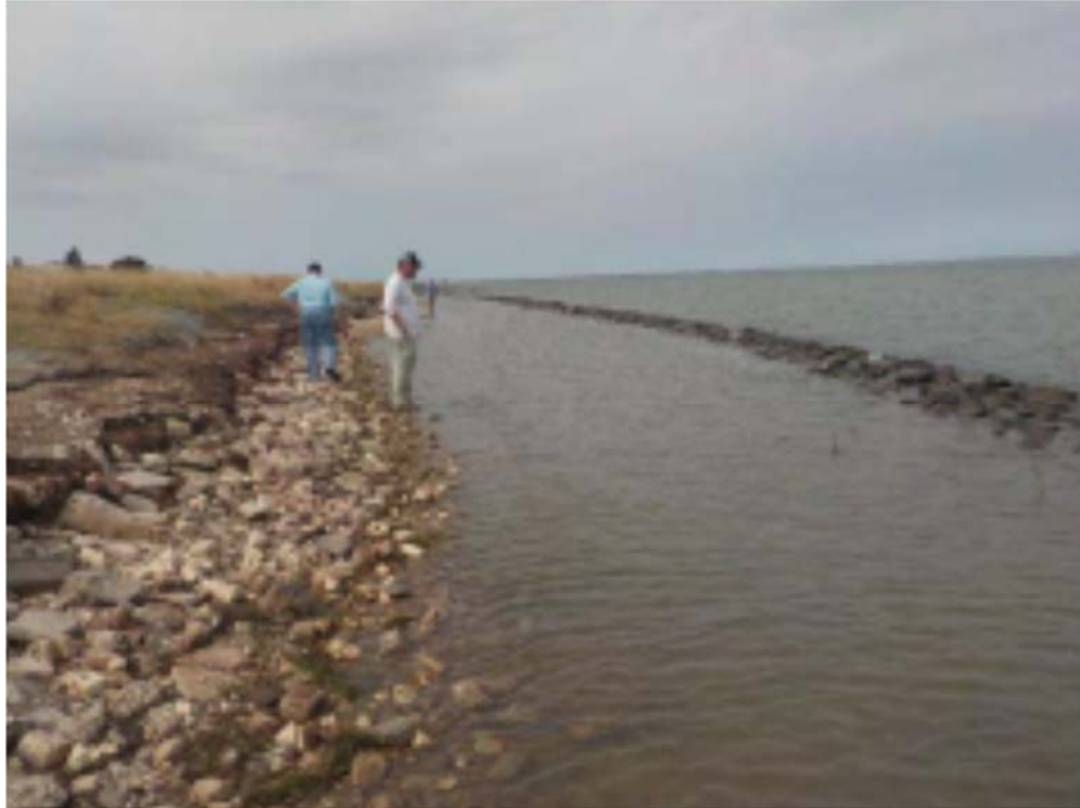
Figure 4.4.4 Post-construction Shoreline Erosion observed as observed in December 2015 (Belaire Environmental 2015)
