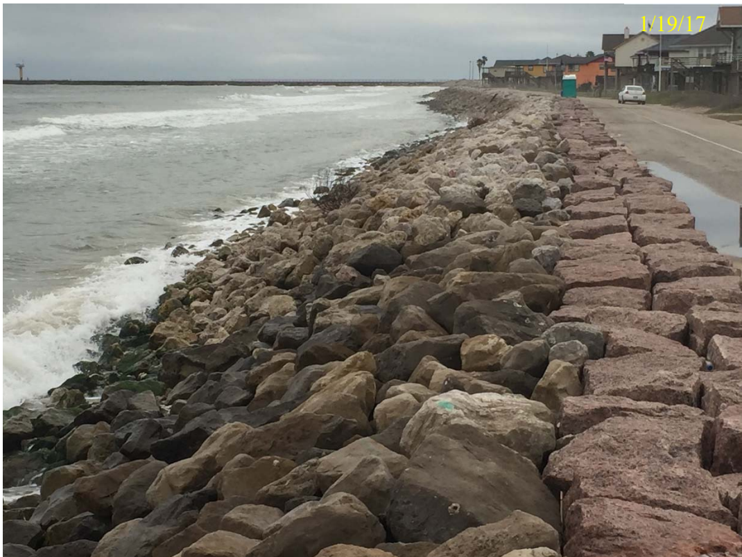
Figure 3.3.6 Eastward (top photo) and Westward (bottom photo) View at East End of Revetment Repair, Present Conditions (1/19/17)
