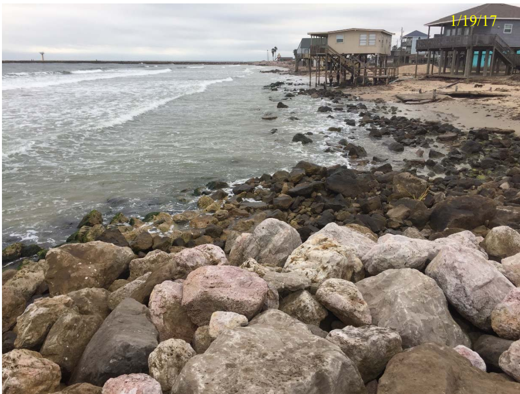
Figure 3.3.7 Eastward (top photo) and Westward (bottom photo) View at West End of Revetment Repair, Present Conditions (1/19/17)
