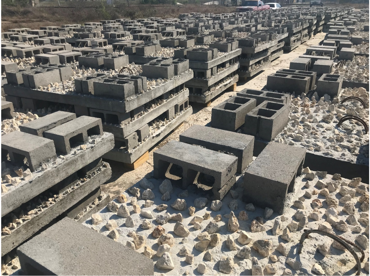
Figure 3. Low relief reef plates completed and staged in Freeport for trucking to Port Isabel for deployment preparations.
