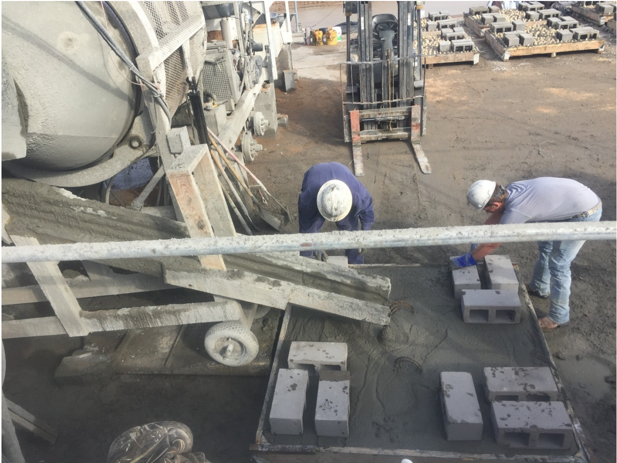
Figure 2. Construction of the low relief reef plates for the Rio Grande Valley Nearshore Reef Site (PS-1105).
