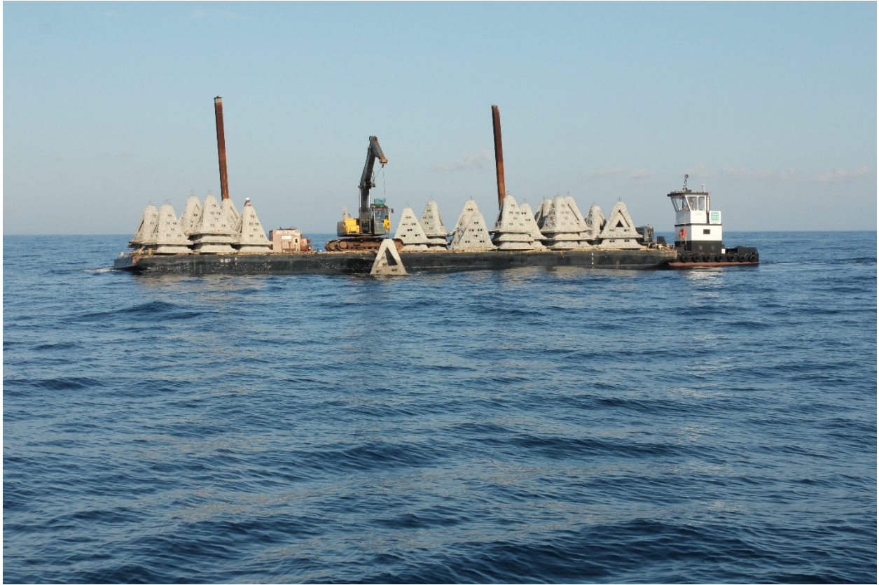
Figure 7. Deployment image of the mid relief pyramids being placed in the Rio Grande Valley Nearshore Reef Site (PS-1005) on 23 August 2018.
