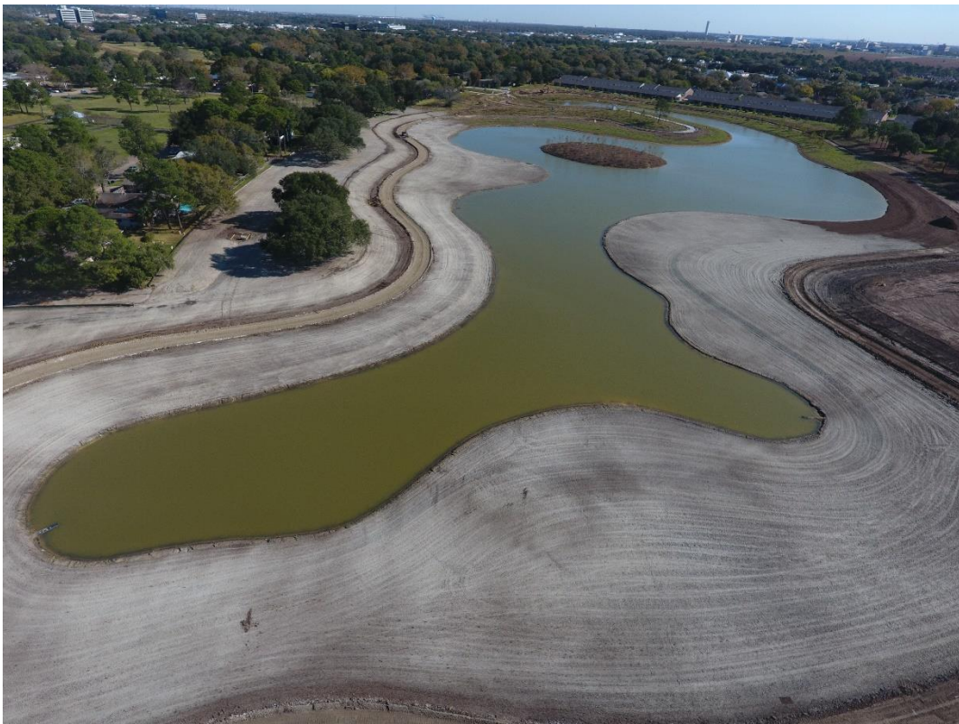
Figure 14. Phase 1A through C facing east after land bridge was removed from habitat island.
