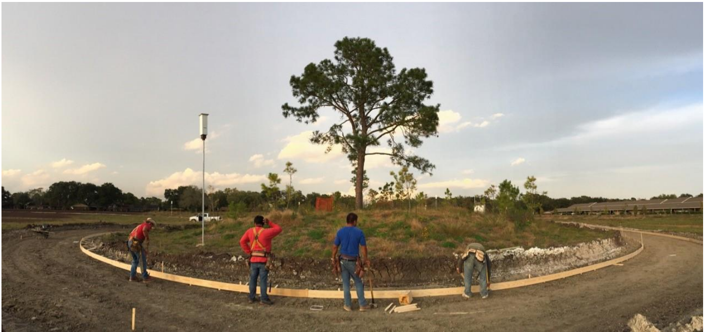
Figure 28. Trail construction around Phase 1A with bat box installed by a boy scout as a separate project.
