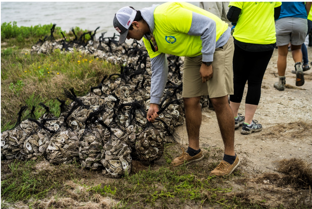
Figure 12. Placing filled shell bags along the shoreline at a community-based restoration event at Goose Island State Park.
