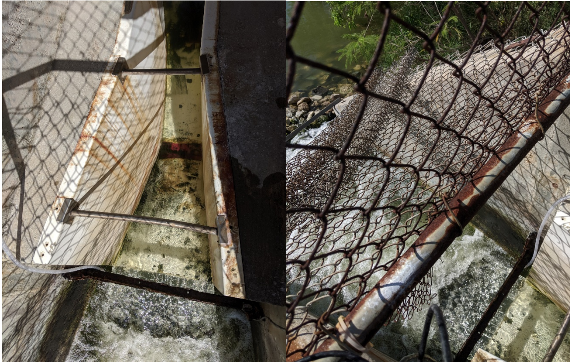
Figure 4. Photos of the Portland WWTP effluent outfall from the front (left), and from the top (right).
