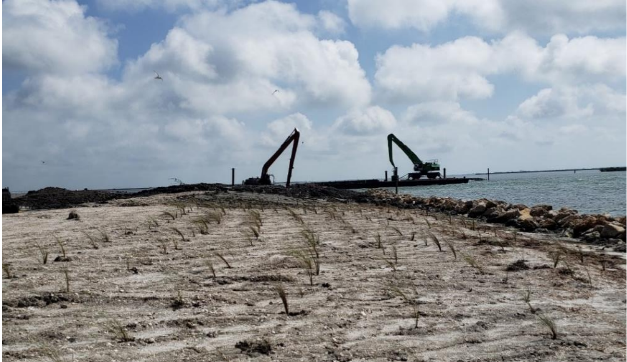
Figure 20. Site 2: levee face comparison, pre-Hurricane Hanna.
