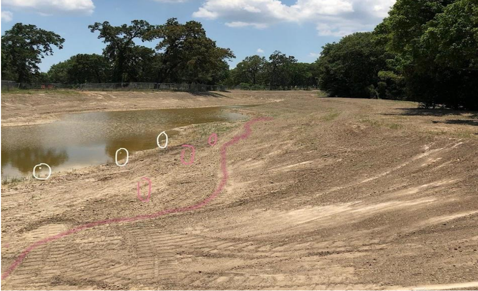
Figure 15: Photo depicting the pin flags marking the wetland planting zone prior to the water test.
