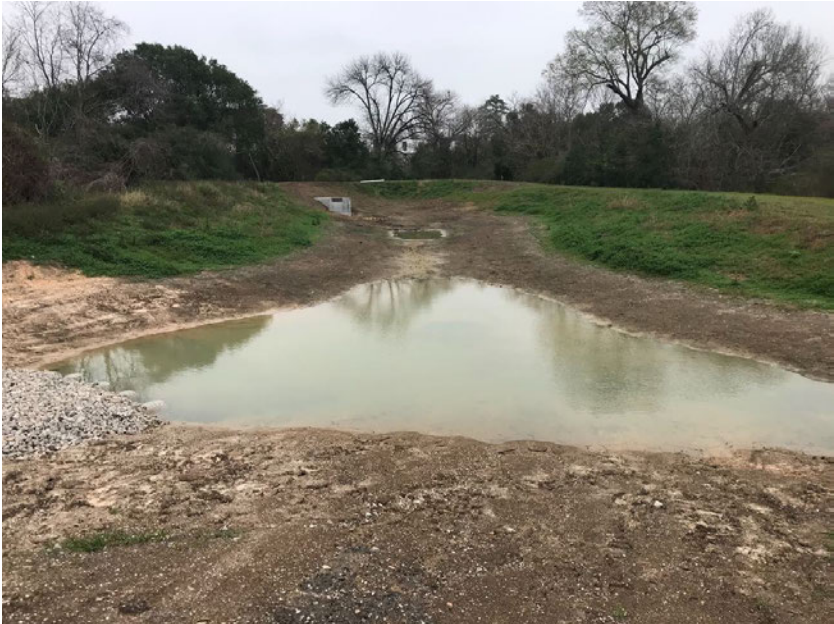
Figure 12: Looking northeast from the 4 culvert pipes that connect basins 2 and 3 toward the outfall structure connected to Sims Bayou.
