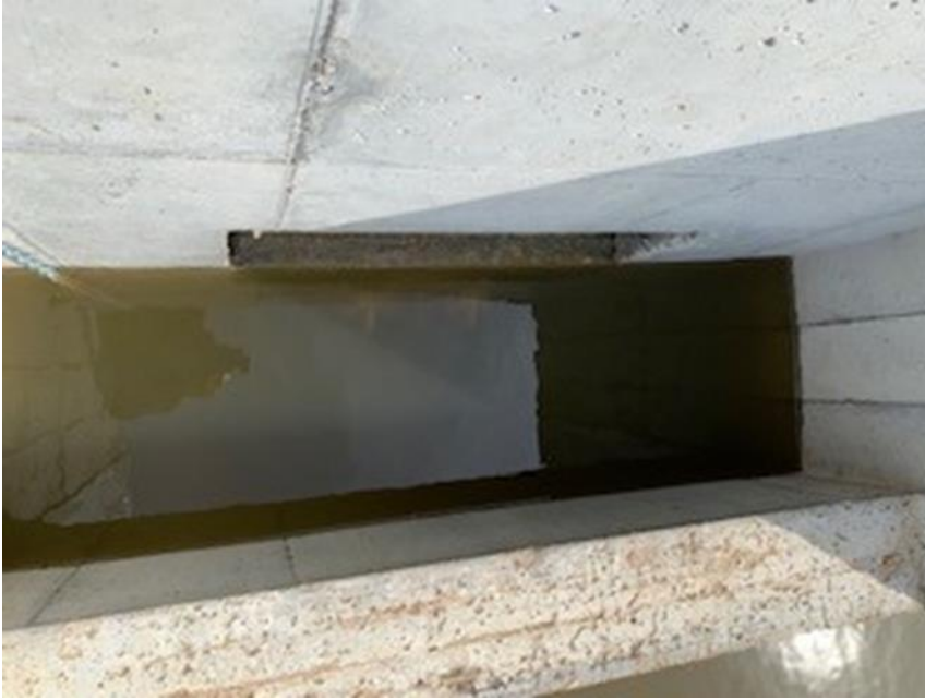
Figure 13: Looking down into the first section of the outfall structure you see the control level opening and the overflow wall.
