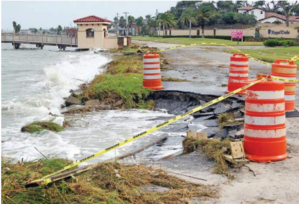
Figure 3. Photo taken by Rockport Pilot showing significant road damage from Hurricane Hanna.
