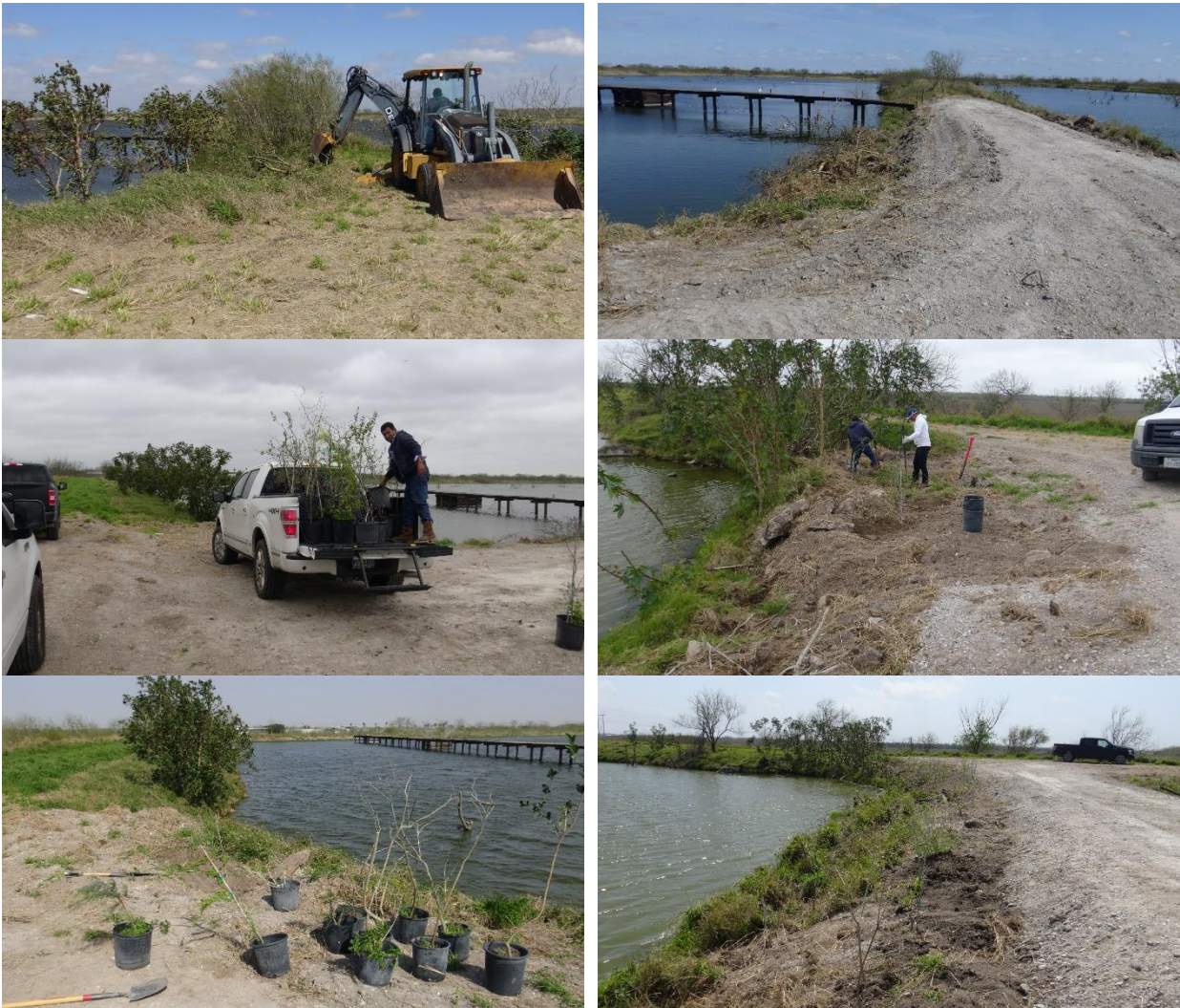
Site preparation, planting, and after planting results on the Phase III wetlands
