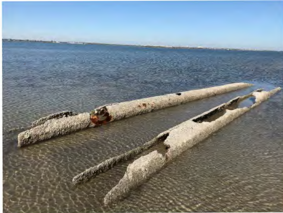
Photo 9: Deteriorating pipes on north side Tern Rookery Island.
