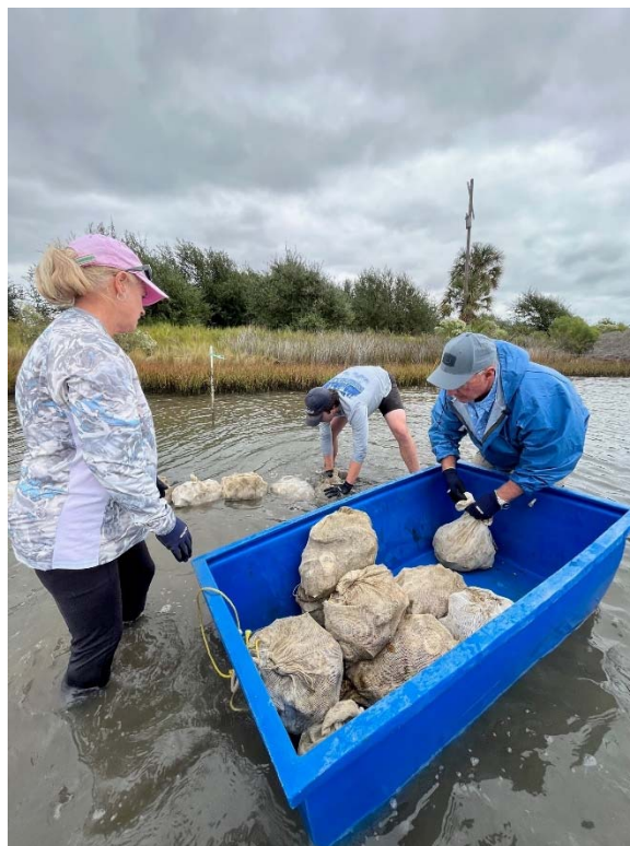
Figure 13. Volunteers placing oysters and recycled shell onto Sweetwater Lake Oyster Shell Breakwater (Fall 2022)
