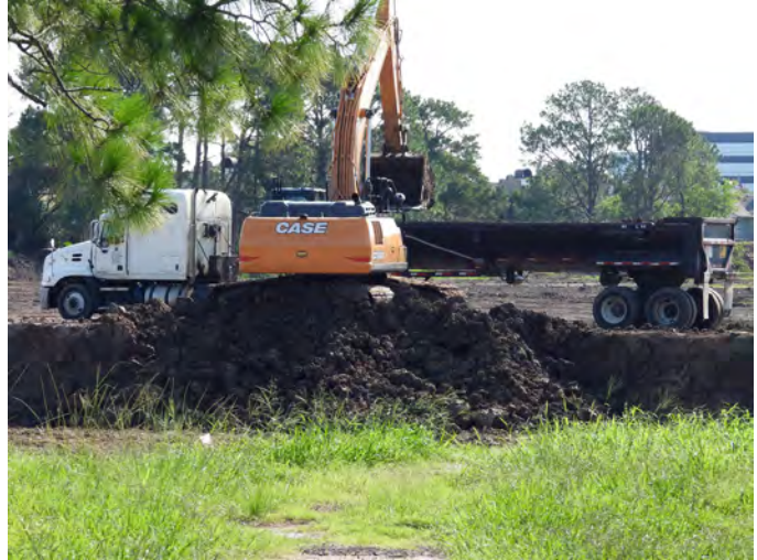
Figure 23: Hauling excess topsoil from excavation off property. Photo courtesy of Jason Miles.
