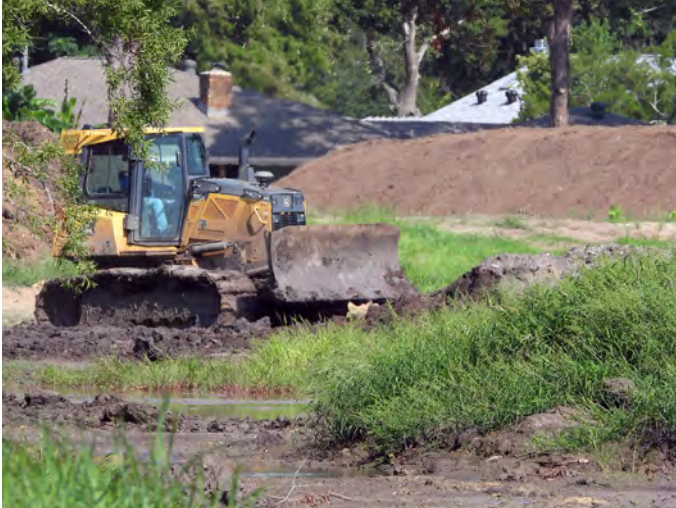
Figure 22: Excavation of Phase 5 of Exploration Green. Construction photos courtesy of Jason Miles.
