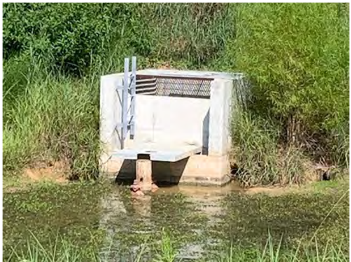
Figure 24: Outfall structure at Houston Botanic Garden Stormwater wetland at low water level. showing clean out ladder.
