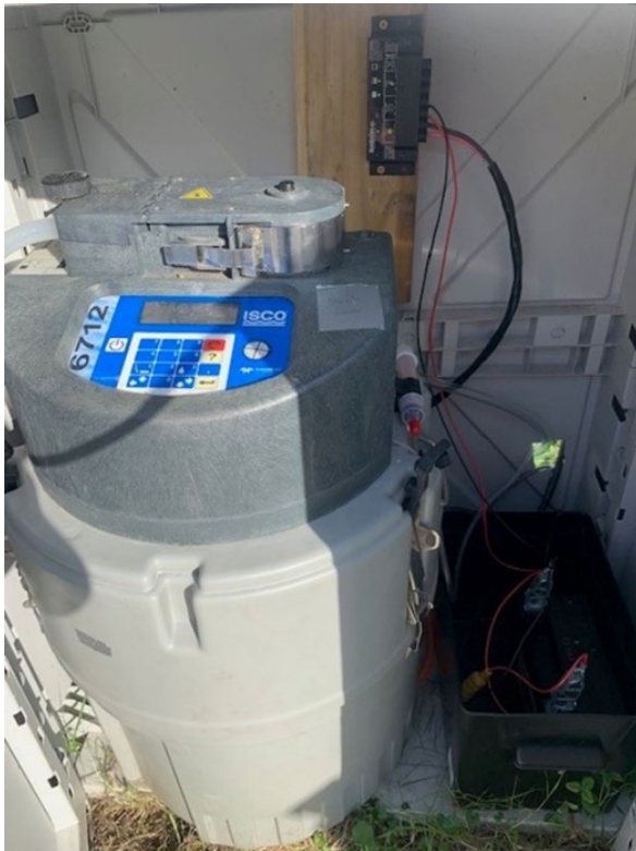
Figure 9 View of equipment inside the box, including solar array wire housing, battery, and sampler.
