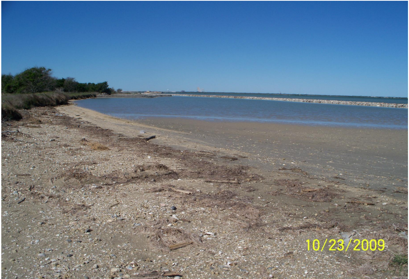
Photo Station 5. Post-construction. East portion of shoreline nourishment and mid to east sections of completed breakwater.
