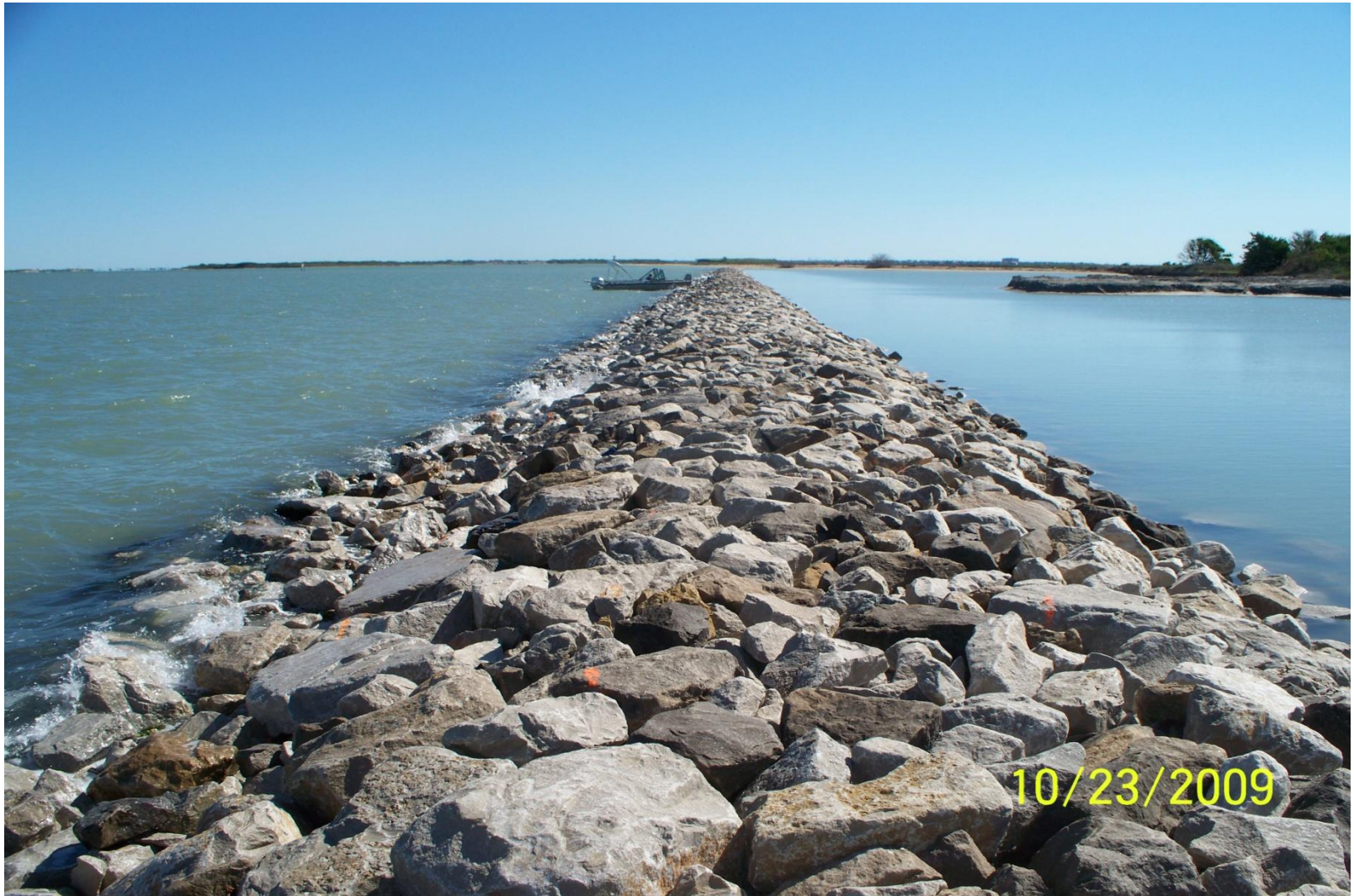
Miscellaneous Post Construction photo. Typical completed breakwater section profile. Looking east along alignment. 10/23/2009.
