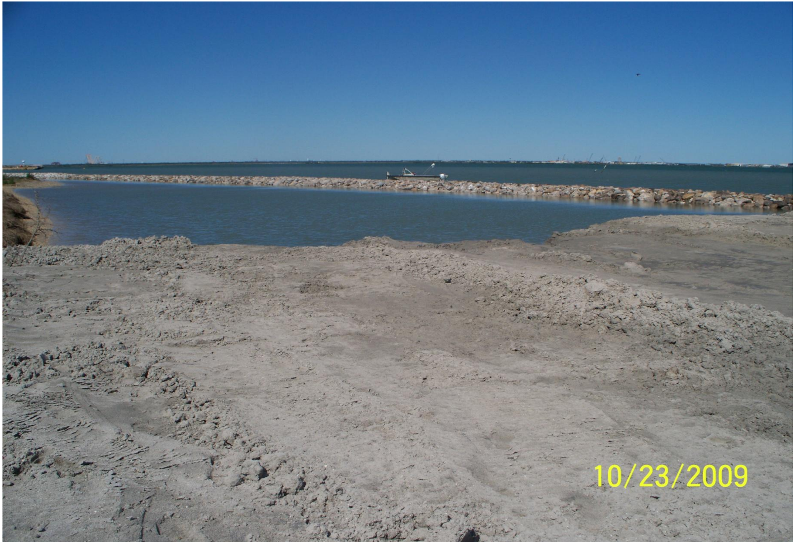
Photo Station 3. Post-construction . West end of shoreline nourishment behind completed breakwater section.
