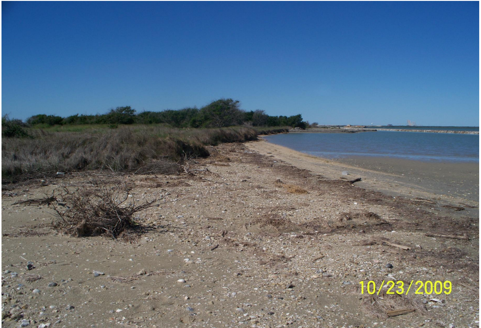
Photo Station 5. Post-construction. East portion of shoreline nourishment in mid distance and completed breakwater to right.
