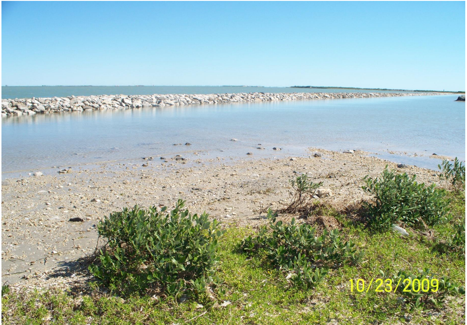
Photo Station 2. Post-construction . Note erosion between pre-construction photo and post construction.
