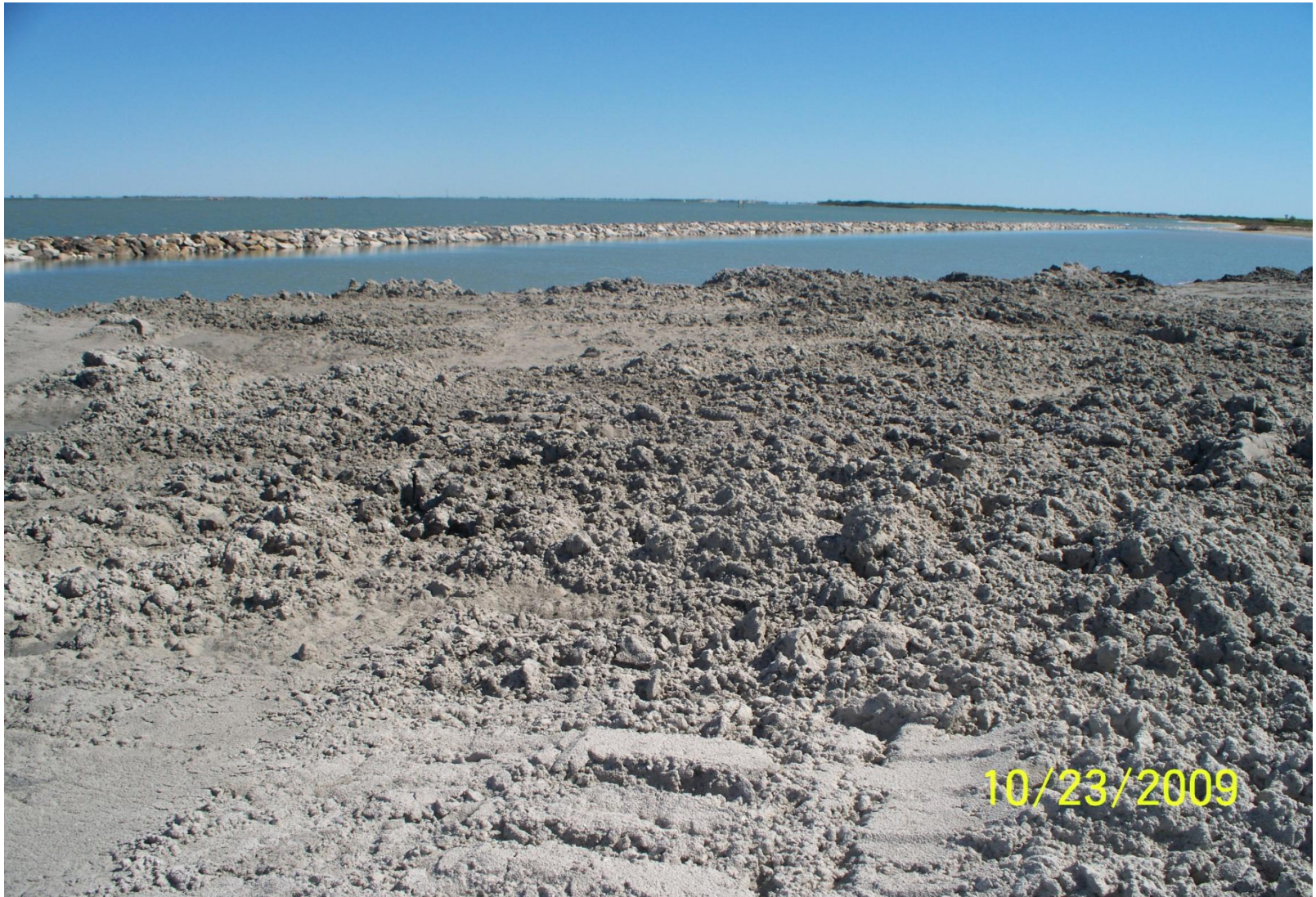
Photo Station 3. Post-construction. View north east along Ship Channel. Shoreline nourishment and breakwater.
