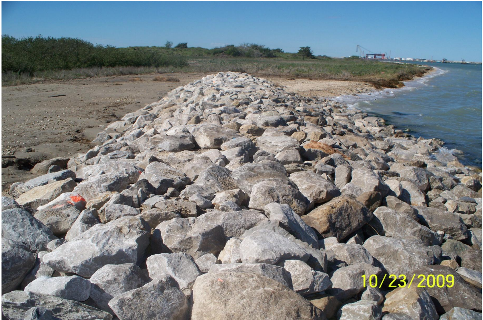
Miscellaneous Post Construction photo. Typical completed revetment section profile. Looking southwestward along alignment. 10/23/2009
