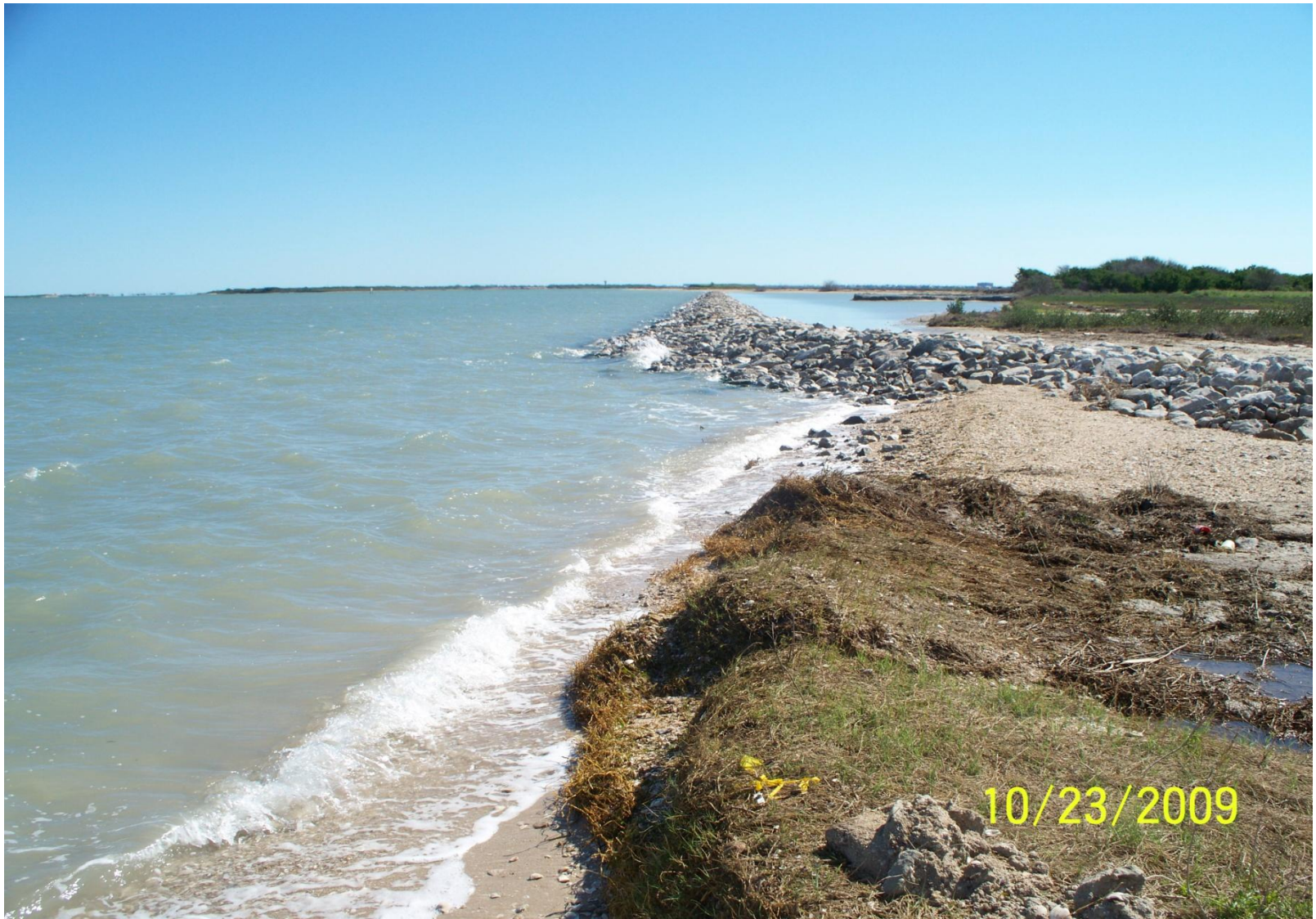
Photo Station 1. Post-construction . View east down alignment of completed breakwater. Note bank erosion compared to July 2009 photo.
