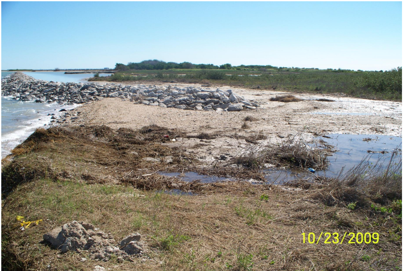
Photo Station 1 Post-construction . View east view toward Photo Station 2. Project revetment section in foreground.
