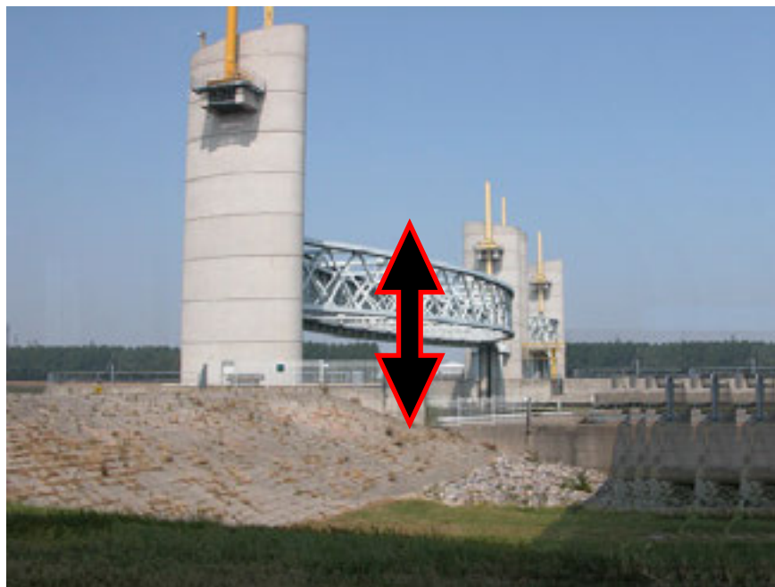
Figure 31 - Typical Vertical Lift Gate
