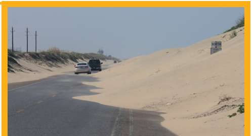
State Park Road 100 overrun by dune sands as natural systems and infrastructure intersect. (Photo Credit: Texas General Land Office)
