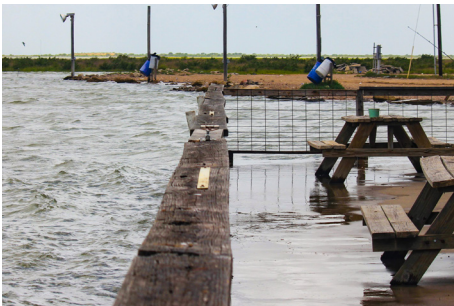
An inundated deck during a highwater event. (Photo Credit: Texas General Land Office)
