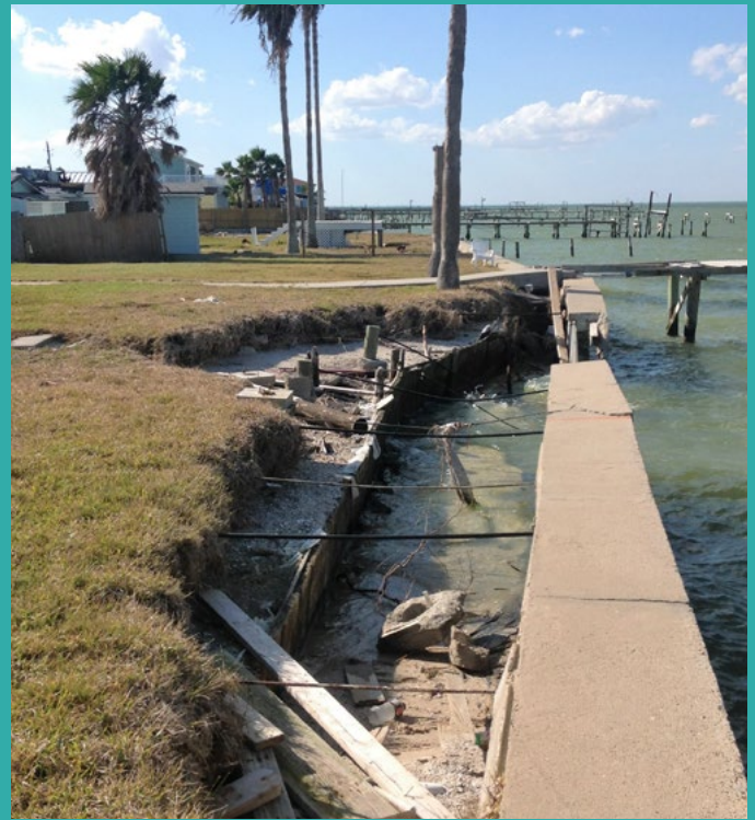
Bulkhead failure (Photo Credit: Galveston Bay Foundation)
