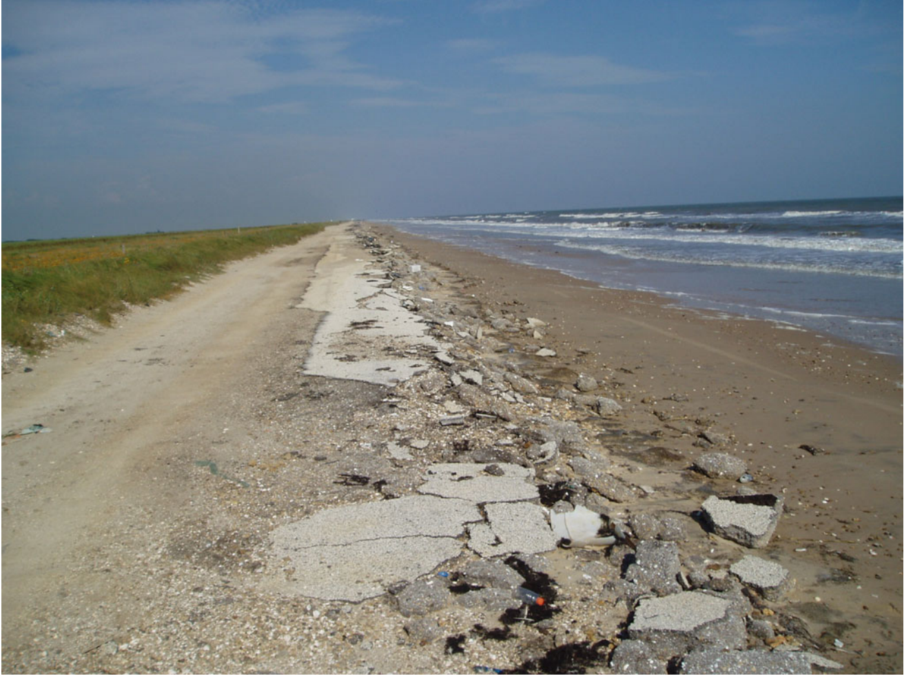
Figure 47. Evidence of Gulf shoreline erosion along the strandplain-chenier system. Photo, taken in October 2006, shows remnants of Highway 87 approximately 6.5 km northeast of High Island.
