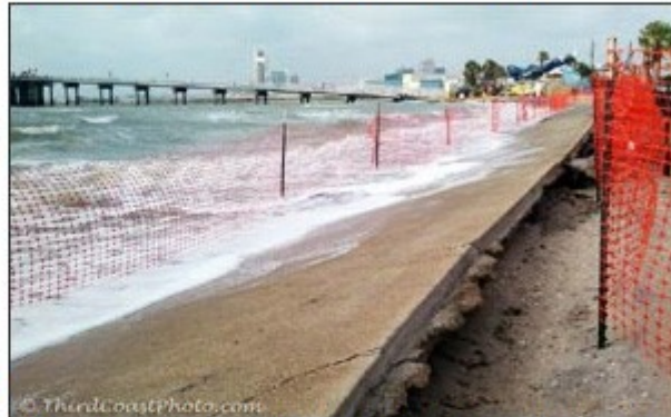
After erosion caused the Beachwalk to collapse, the city secured emergency funding to repair it.
